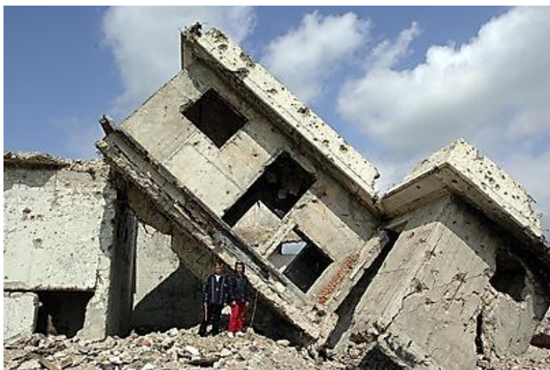
A building damaged in the war in Kosovo. Photo: UN Photo
